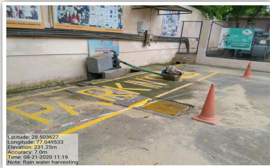
Figure 1: Rainwater harvesting and recharge pits
